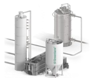
Cascade H_2S Biogas Desulfurization
